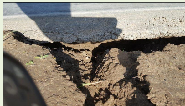
Figure 50: Ground Cracking and Structural Instability Due to Soil Settlement
