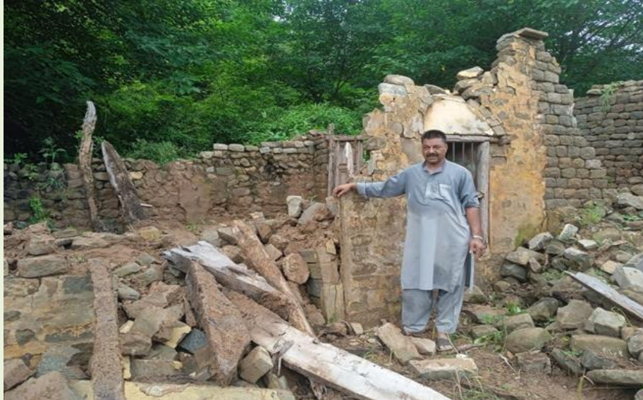
Figure 46: Structural Failure of an Aged Residential Unit in Mirpur Due to Lack of Maintenance
