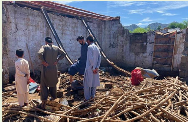
Figure 30: Roof Collapse in Lyari, Karachi due to Heavy Rainfall
