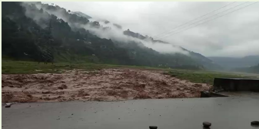
Figure 45: Road and Riverbank Erosion in Bagh Due to Absence of Stabilization Measures
