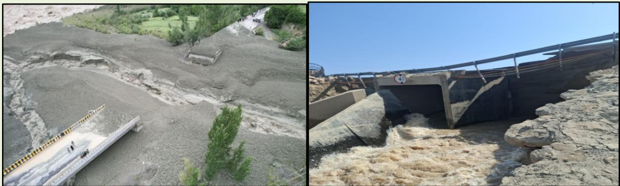
Figure 56: Structural Impacts of Sedimentation and Debris Load on Bridge and Culvert Systems
