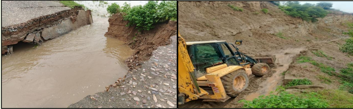
Figure 57: Road and Infrastructure Damage Caused by Soil Erosion and Landslide Deposition
