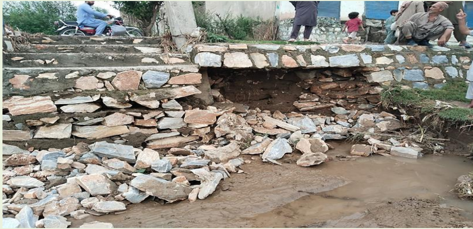
Figure 3: Structural Erosion and Material Degradation in Swabi Following Flash Flood
