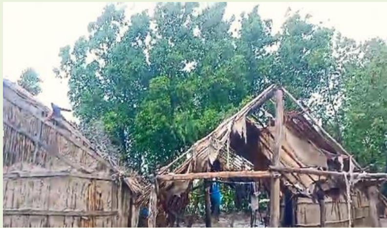
Figure 31: Mud and Thatch House Damage due to Flash Flooding Triggered by Intense Monsoon Rainfall
