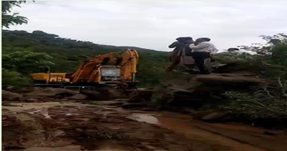
Figure 44: Landslide in Sudhnoti Triggered by Heavy Rainfall and Absence of Retaining Structures
