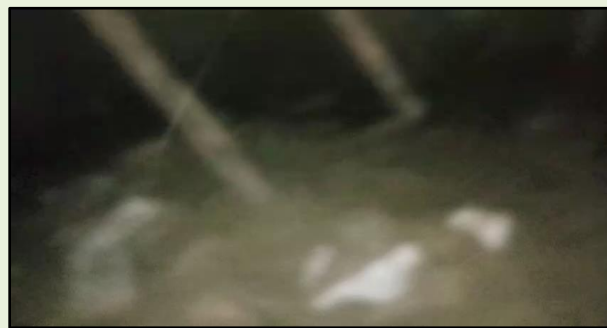
Figure 51: Water Accumulation and Structural Deterioration Due to Inadequate Drainage Planning
