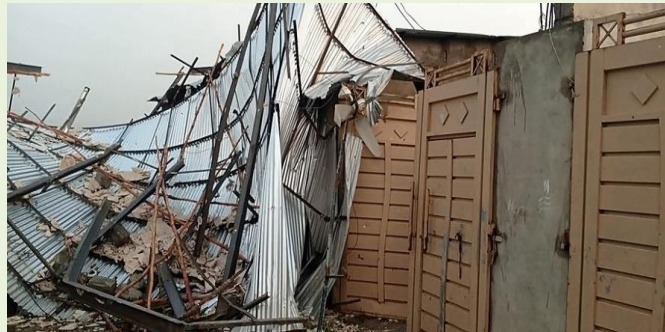
Figure 23: Roof Collapse in Muslim Bagh due to Heavy Rainfall
