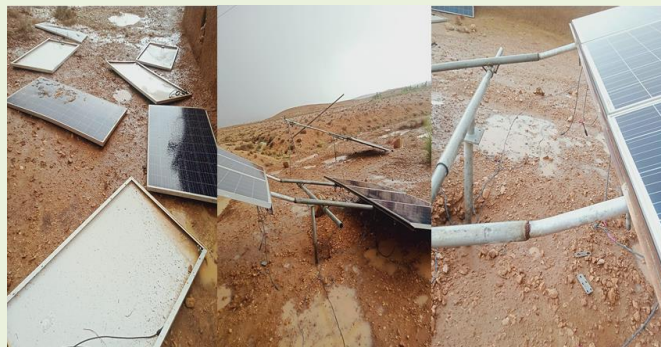
Figure 22: Solar Infrastructure Damage due to Heavy Rainfall
