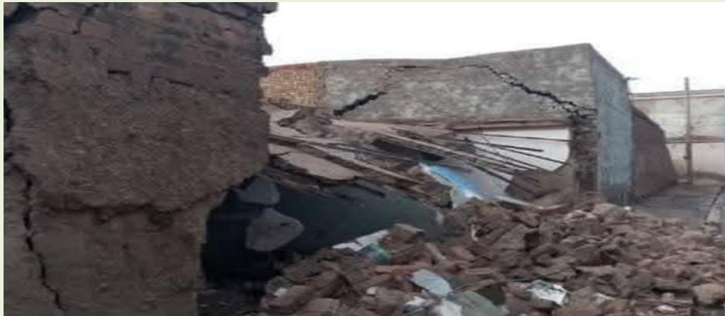
Figure 9: Structural Collapse of Houses
