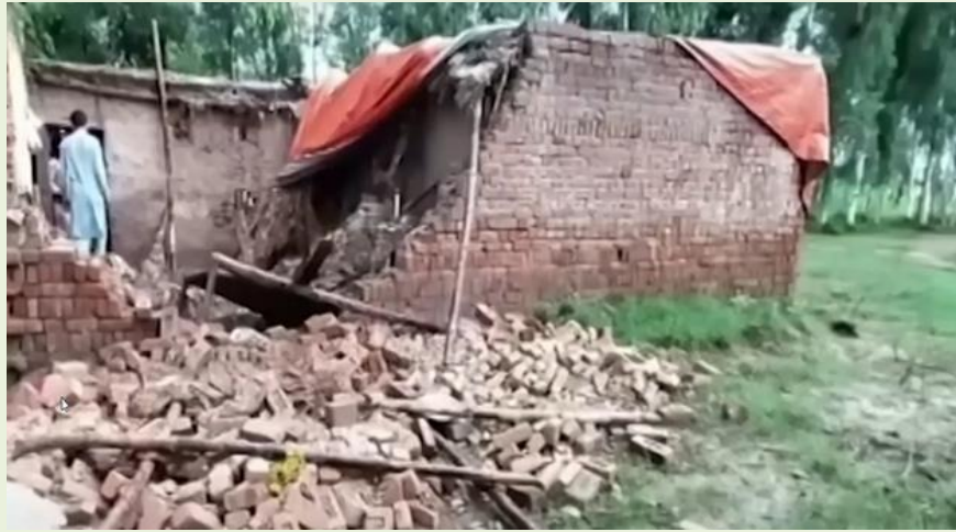
Figure 13: Structural Collapse of Residential Houses in Sargodha Due to Poor Construction Practices
