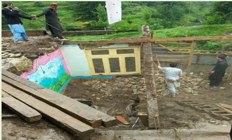
Figure 6: Roof Collapse Due to Rainwater Accumulation
