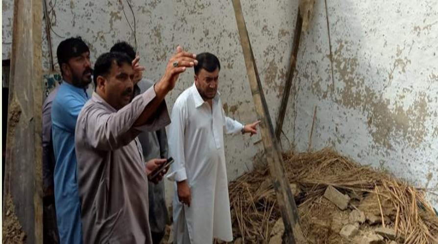
Figure 20: Roof Collapse in Harnai due to Intense Rainfall
