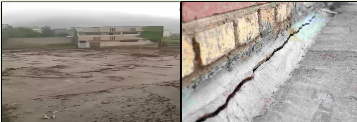
Figure 52: Foundation Failure and Structural Cracking Caused by Poor Drainage and Soil Instability
