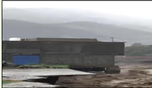
Figure 47: Structural Instability Caused by Foundation Soil Erosion
