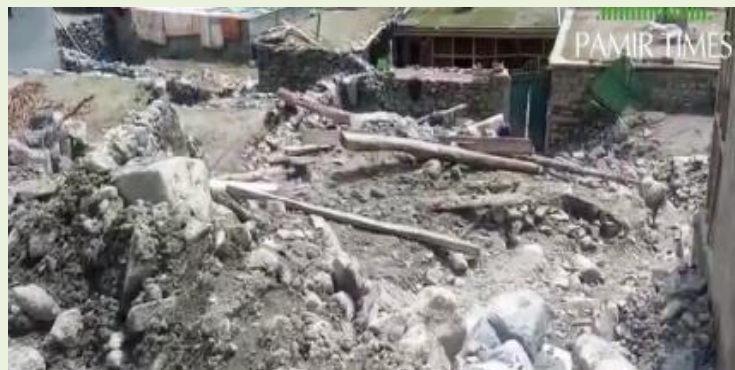
Figure 37: Structural Collapse of Residential Houses in Gilgit Following Flash Flood
