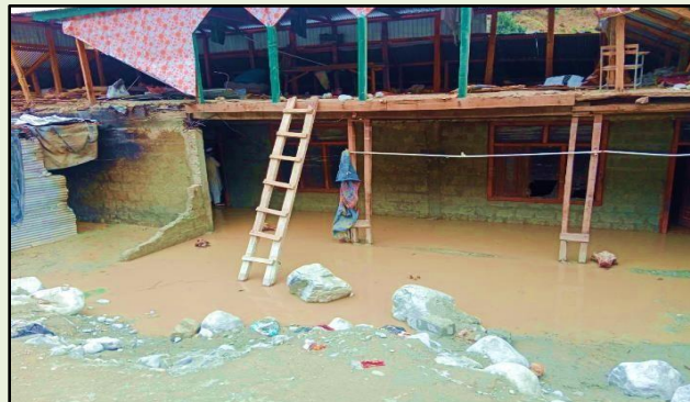
Figure 48: Waterlogging Around Residential Structures Due to Blocked Drainage Systems
