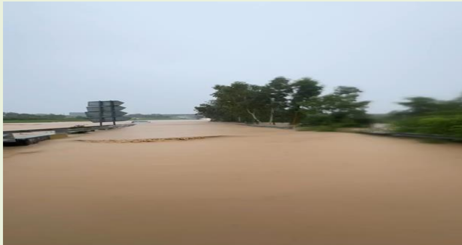
Figure 12: Flooding and Water Accumulation on Motorway Due to Blocked Drainage Network
