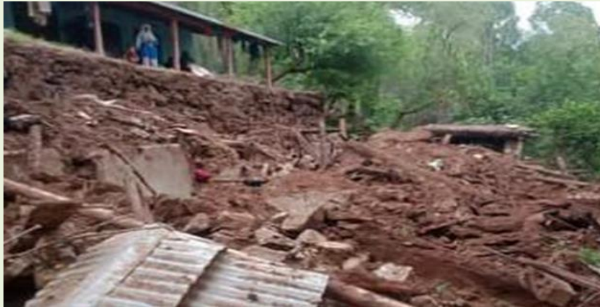
Figure 41: Structural Collapse of Residential Buildings in Sudhnoti Due to Weak Design and Materials
