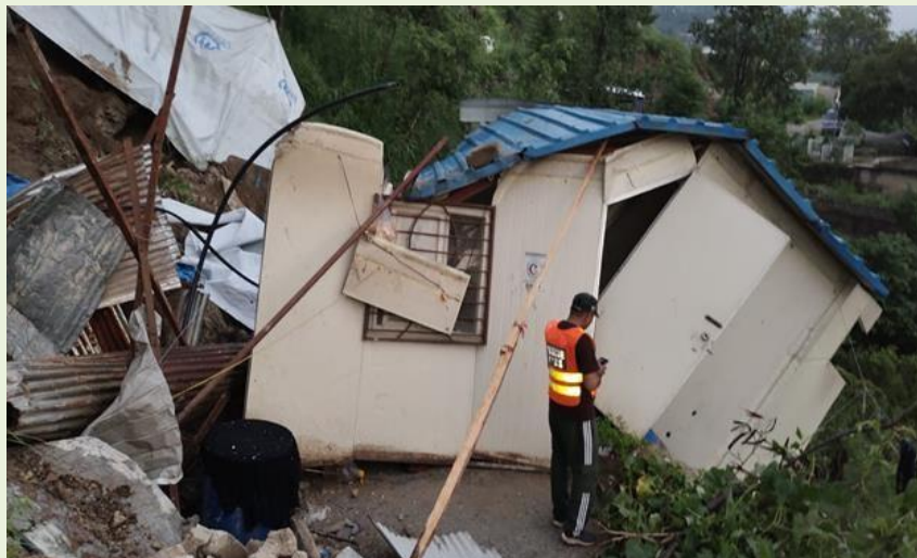
Figure 42: Structural Collapse of a Residential Unit in Muzaffarabad Due to Poor Site Selection
