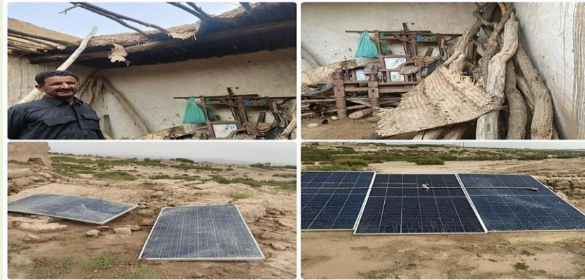
Figure 21: Roof and Solar Infrastructure Damage in Surab due to Heavy Rainfall
