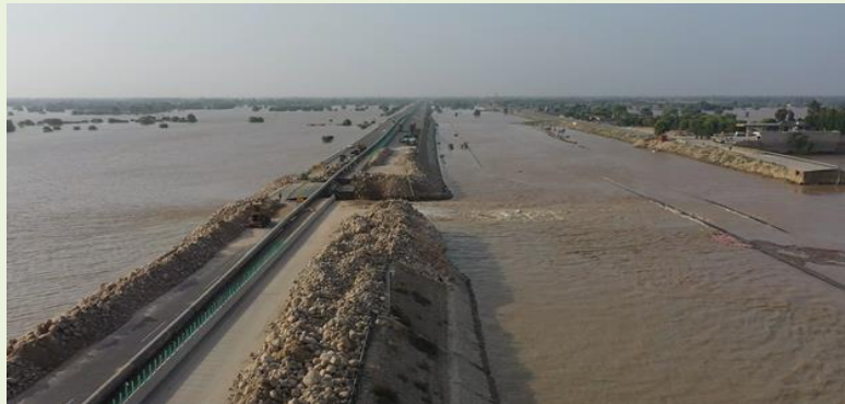
Figure 17: Flood-Induced Erosion and Embankment Collapse on M-5 Motorway, Multan
