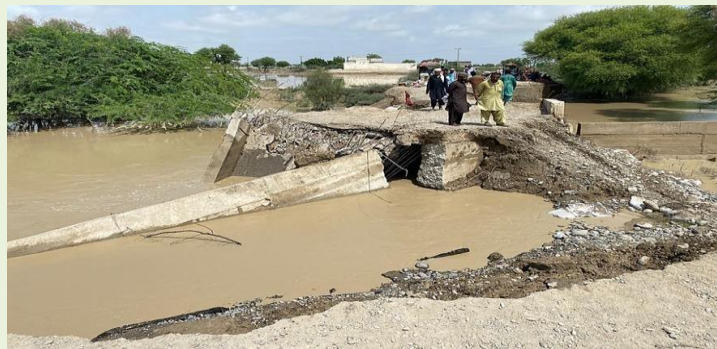
Figure 24: Bridge Washed Away in Lasbela due to Severe Flashflood
