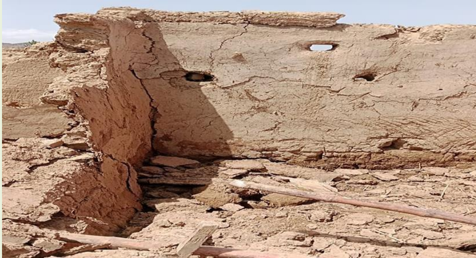
Figure 19: House Damage in Musakhail due to Intense Rainfall
